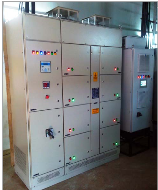
The hybrid PFC solution installation at site (left side detuned PFC system, right side Active Harmonic Filter)
